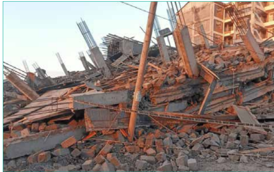
Another building that collapsed while under construction near Nairobi
