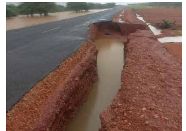
The ongoing heavy rains have caused havoc in many parts of the country making roads impassable. This is a section of Thika-Garissa Road.
