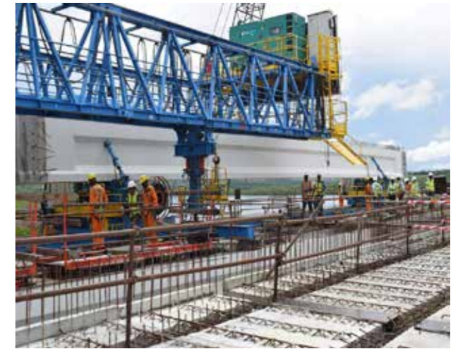
Installation of the last girder in the Mombasa Port Area Development (MPARD) Package 2 Road project at the 1.4km Mteza Bridge this November.
