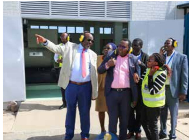
Kenya Airports Authority Board of Directors, led by Chairman Caleb Kositany (pointing) inspected the newly upgraded power backup generator system at JKIA.
