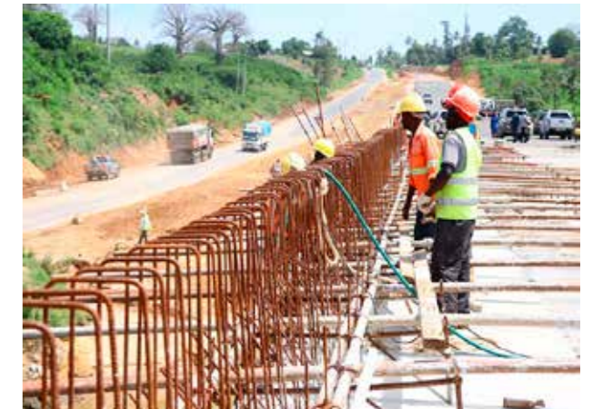
The Bagamoyo-Tanga-Horohoro/Lunga Lunga-Malindi Road, a road connecting Kenya and Tanzania that was commissioned under the East African Community, is on course.
